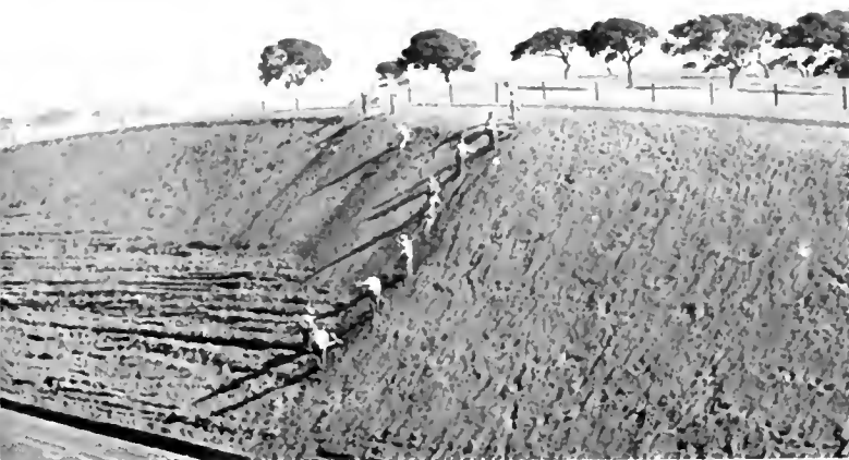
Raking top soil down—Improved appearance of cuts after covering would justify this method if no other factors were involved
